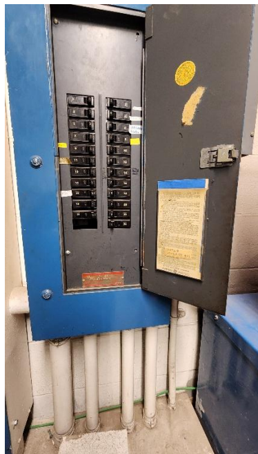
Photo 11: Maintenance Room Panel #1 open
