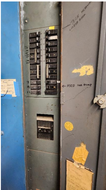
Photo 15: Maintenance Room Panel #3 open
